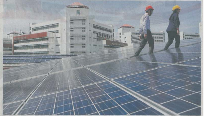
Rooftop solar panels are installed at Thammasat University, Rangsit campus. TANAPHON ONGARITTRAKUL
