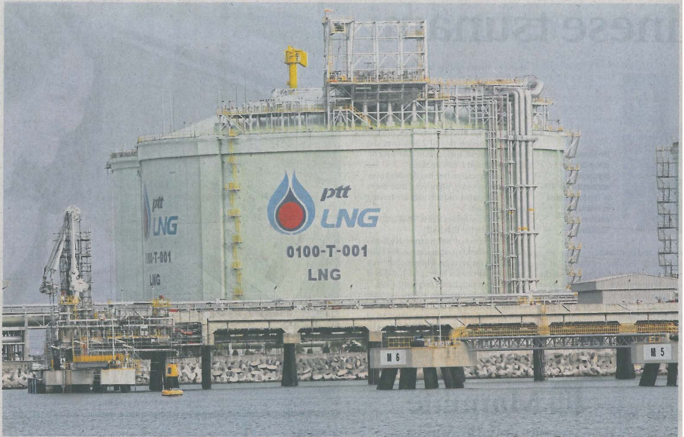
PTT's LNG terminal at Map Ta Phut industrial estate in Rayong province has a capacity of 10 million tonnes, but uses only half that figure. APICHAART JINAKUL
