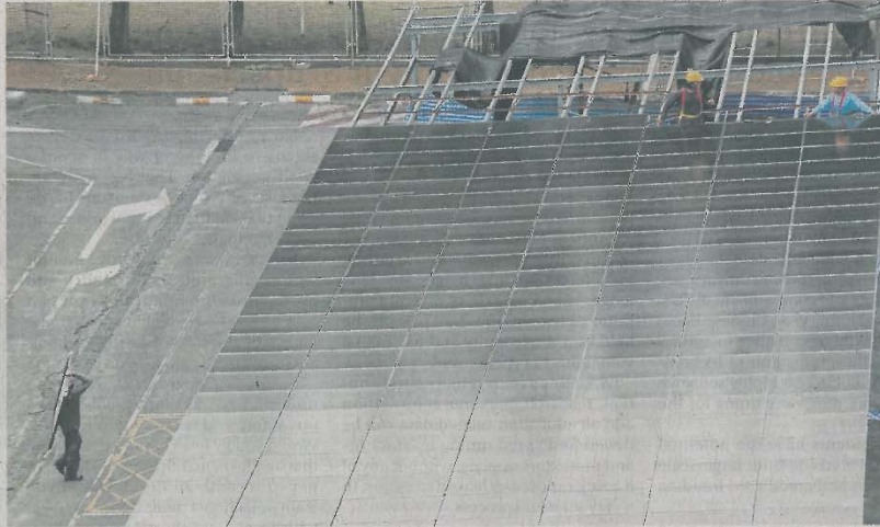
Workers install solar panels. Egat is keen on developing on-site power generation via solar rooftop at industrial estates to promote the smart grid. CHANAT KATANYU
